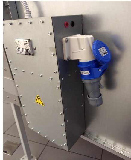
Line filters box: AC and DC input
